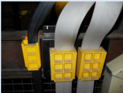
Intricate and difficult to clean surfaces where dust can collect
