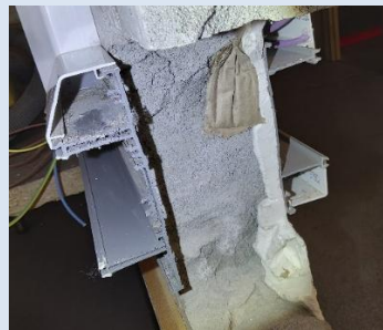
Conduits which have been unsealed or exposed to the removal environment
