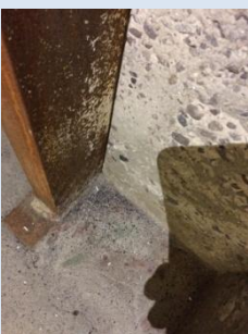
Blast media within cavities and edges adjacent to areas blasted
