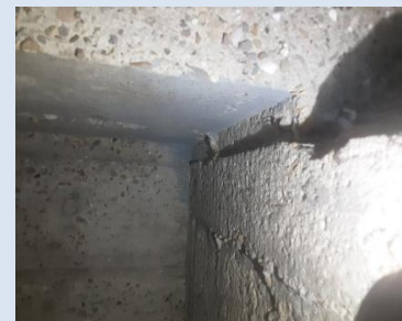
Incomplete removal of encapsulants in difficult to reach alcoves / corners
