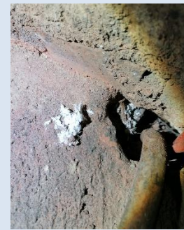
Small openings in floors/walls/ ceilings especially where services penetrate
