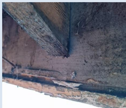
Small gaps between timber structures or finishing surfaces
