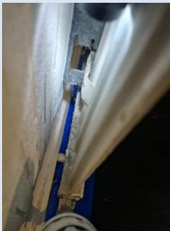
Narrow gaps behind fixed equipment such as wall mounted radiators
