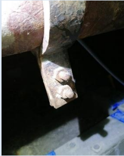
Difficult to clean surfaces like nuts and bolts
