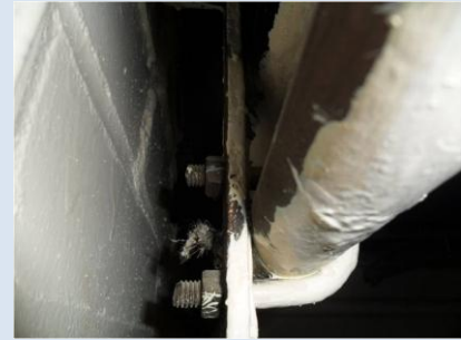
To the rear of pipes especially adjacent to brackets or close to walls & ceilings
