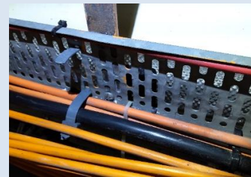
Cable trays, especially beneath unclipped cable bundles
