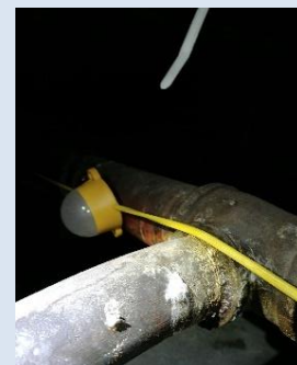
Rough plant surfaces where insulation or cleaning materials can easily be snagged
