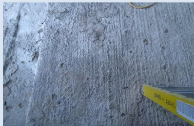
Porous floor or wall surfaces where contamination can collect in the depressions
